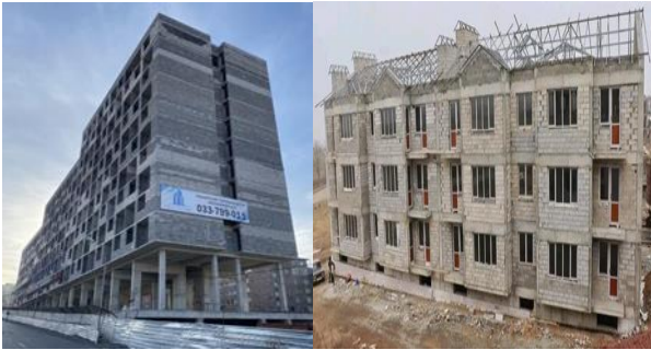
Figure 1. Examples of illiterate construction currently going on in Armenia
